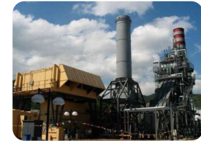
Gas Turbine Control
